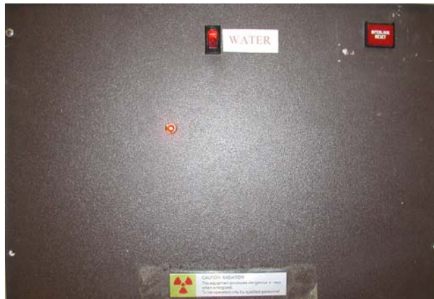
Fig. 2. Water and interlock switches.
